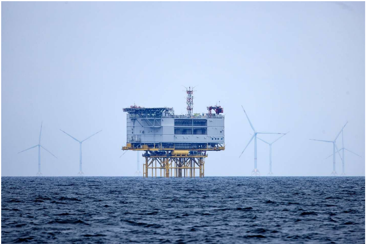
Picture: Baltic Eagle Offshore Substation (HVAC) from Elia Group.
